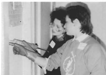
Shannon and Cheryl working at caulking walls. It didn't take long to learn the rhythm.
